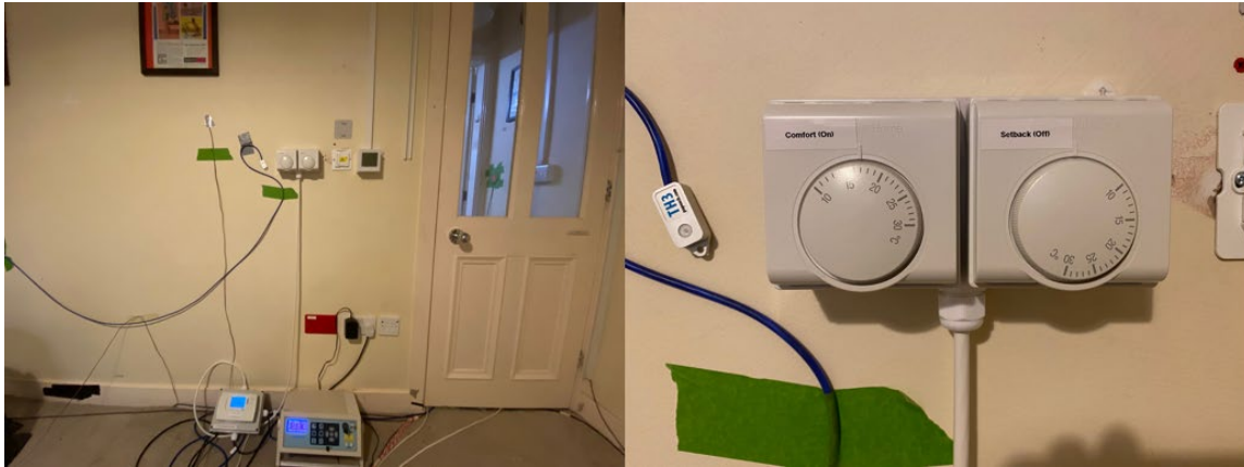
Figure 1. Thermostatic controllers on the living room wall (right thermostat provides setback control)
