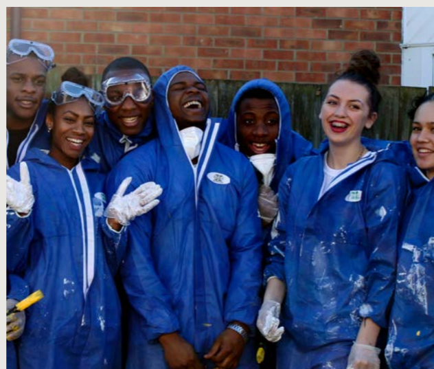
Young people repairing the Selby Centre in Tottenham as part of the Volunteer It Yourself project
